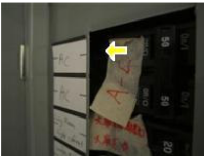
5.1 Picture 1 wide space - safety issue
