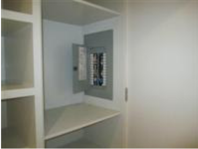
5.6 Picture 1 does not meet access clearance requirements
